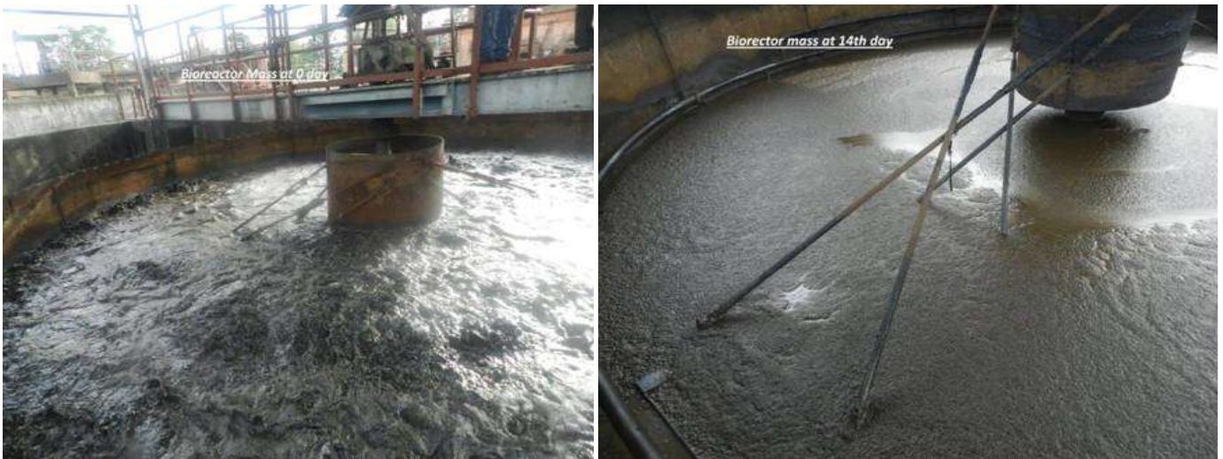
Bio-remediation facility of BGR
